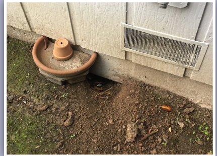
A hole beneath foundation is evidence of a skunk burrow
