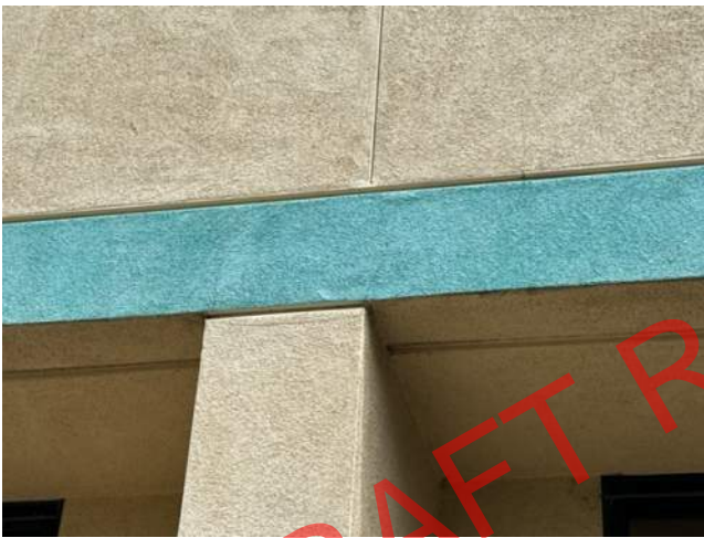
Cracks at wing wall between Windows 2.08 & 2.09. 4102_NBL01_131
