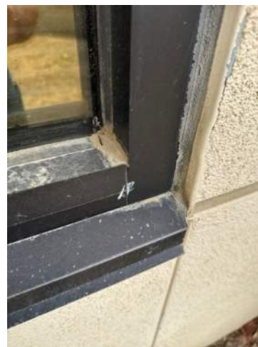
Window 1.11 – Cracked sealant at joint. 4102_NBL01_104
