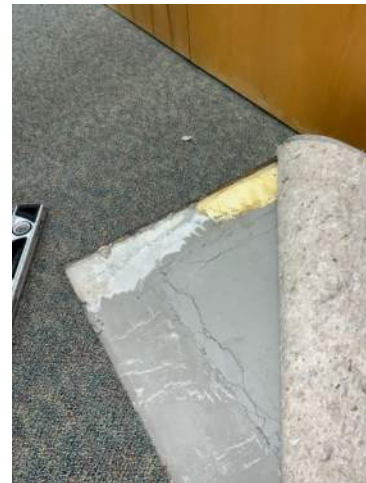
In-situ condition under carpet. 1997 addition side (to the right) appears to be higher. 4102_GEP01_173
