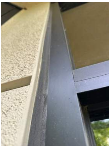
Window 1.09 – Cracked sealant at joint. 4102_NBL01_088
