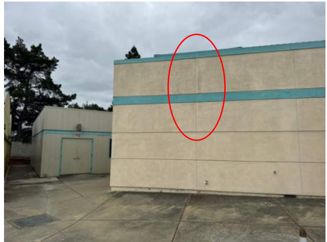
Staining at exterior walls under parapet cap coupling brackets. 4102_NBL01_014
