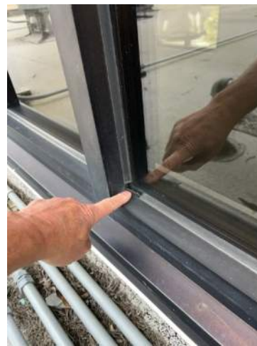
Shrinking at glazing sealant. 4102_GEP01_104
