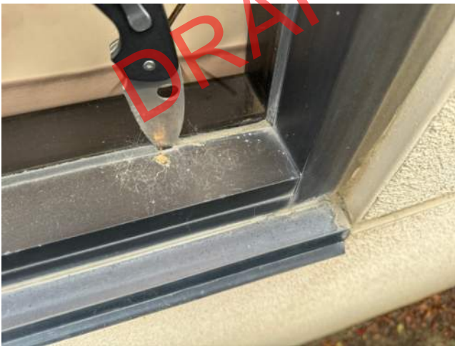
Window 1.20 – Failure of wet-set sealant at glazing.
