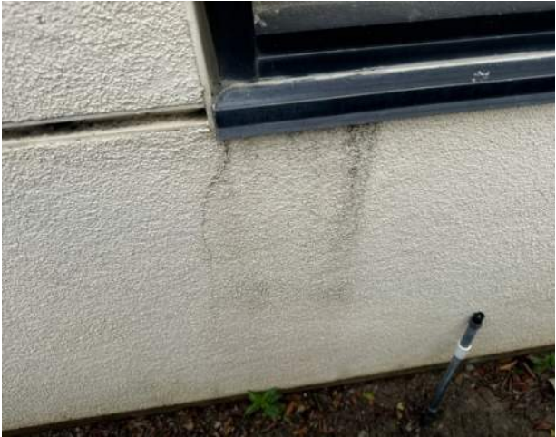
Stucco staining from water discharge under window sill at Window 1.19 – an original window from 1987.
