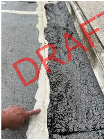
Missing granules at parapet transition. Improper edge sealing. 4102_GEP01_050
