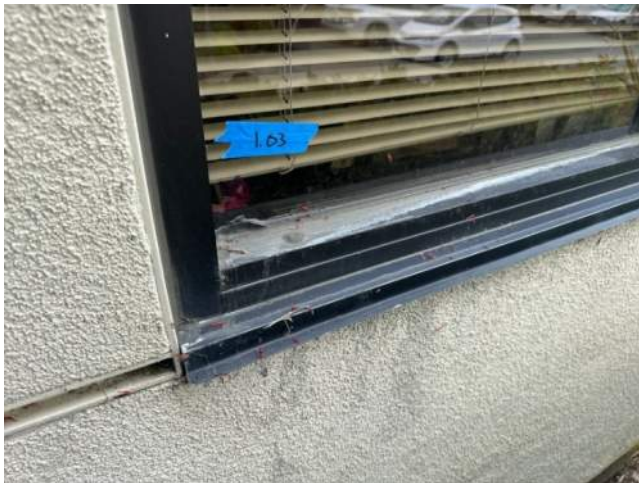
Sill and jamb of original, 1987 window. No visible weep holes. Window 1.03. 4102_NBL01_042
