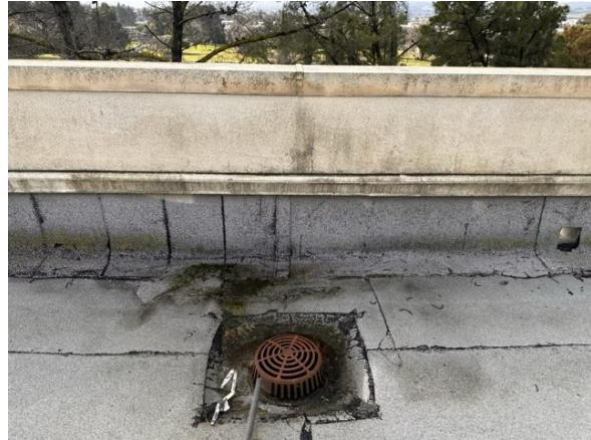
17. Close-up photo of the base flashings. The flashings are suffering from alligatoring, a sign that the membrane is dried out.
