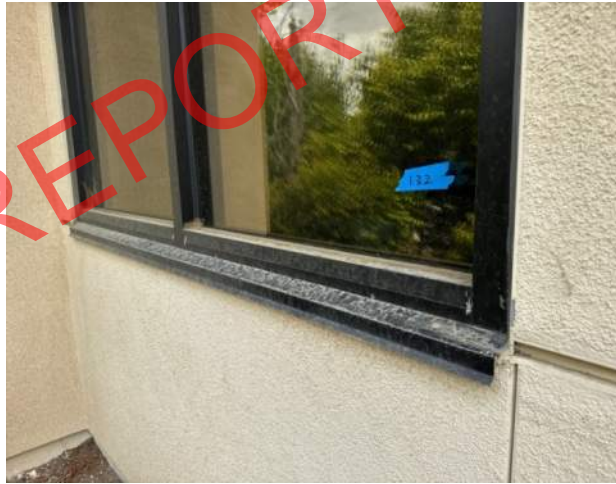
Window 1.32 – Water stippling at base of window. 4102_NBL01_109
