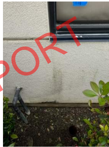
Stucco crack at corner of Window 1.18 4102_NBL01_173
