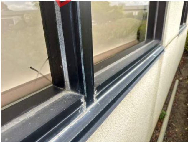
Window 1.19 – reported as active leak. Various joints in window sill have been sealed (white caulking).
