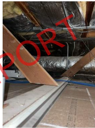
Top of wall bracing for partition at HR Admin Office 4102_GEP01_152
