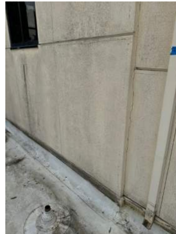
Cracking is stucco at return near Window 2.15 4102_NBL01_245
