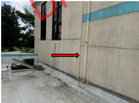
Cracks at small returns in wall at northside of lightwell wall. 4102_NBL01_344
