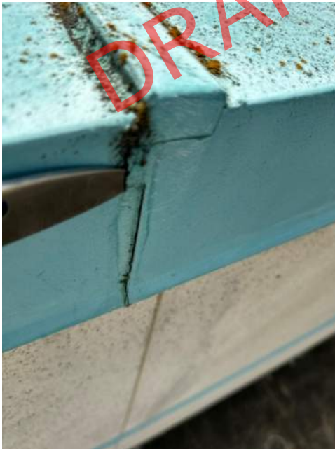
Failed sealant at parapet cap couplers. 4102_NBL01_356
