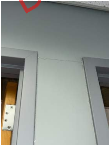
Crack in drywall adjacent to HR admin office door. 4102_GEP01_162
