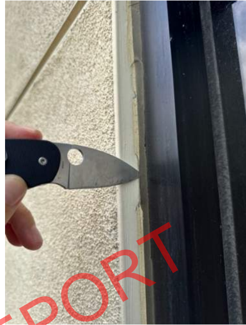
Window 1.20 – sealant failure between window jamb and casing bead.
