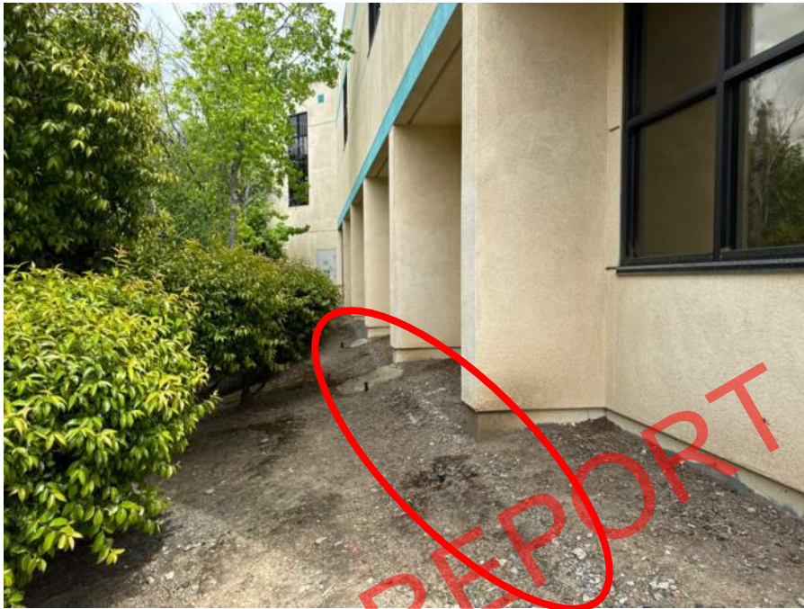
Erosion of soil under drip edges. Also note splash-back at bottom of wing walls.
