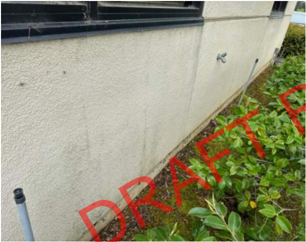
Irrigation Sprinklers adjacent to structure at Windows 1.04 & 1.05 4102_NBL01_058
