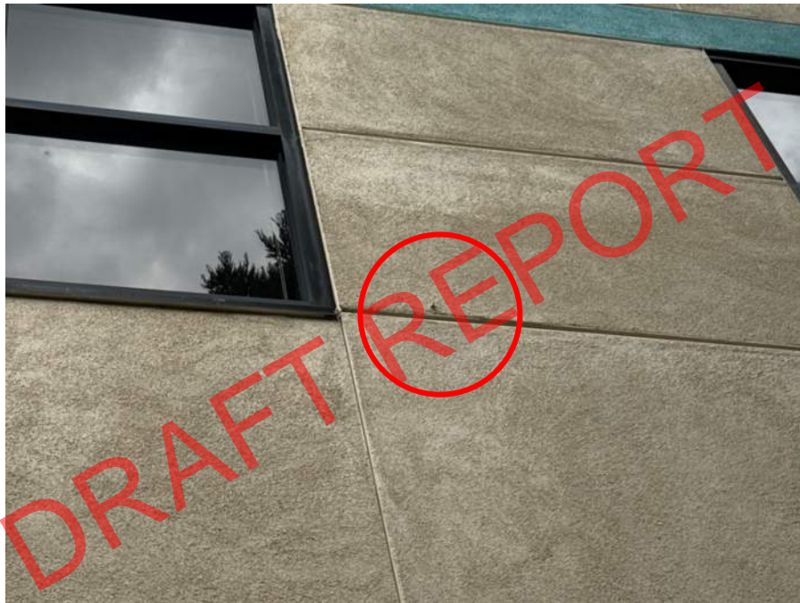
Exposed scaffold tie wire from construction. 4102_NBL01_154
