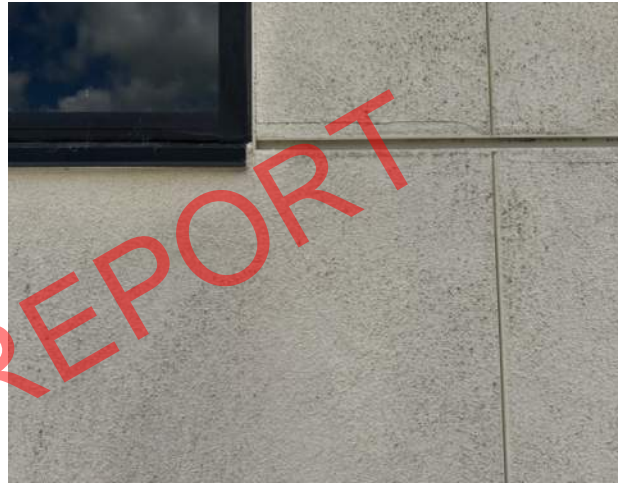
Cracks above and below stucco reveal near Window 2.16. 4102_NBL01_239
