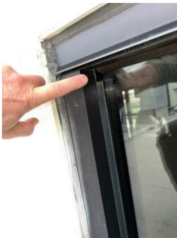
Shrinking at glazing sealant. 4102_GEP01_055
