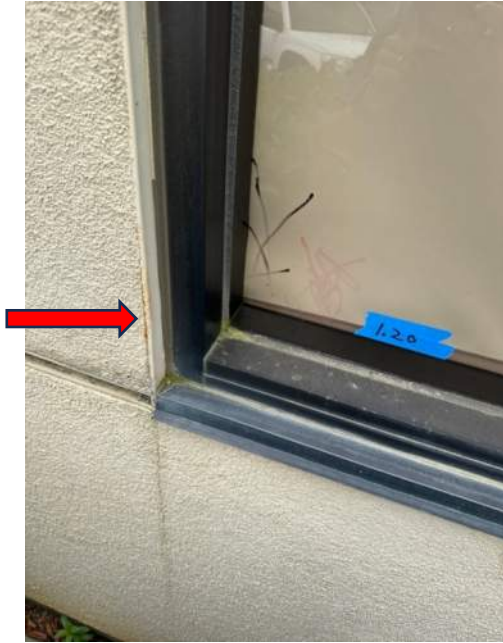
Window 1.20– reported as active leak. Various joints in window sill have been sealed (white caulking). Note rust/corrosion at vertical casing bead.
