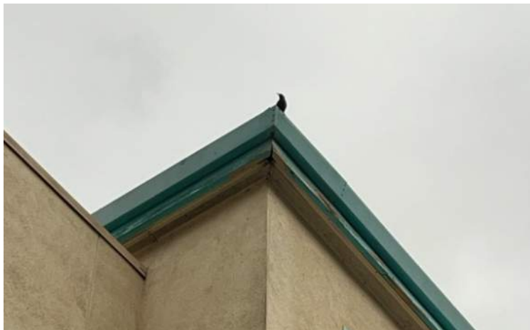
Nesting birds at damaged tower soffits. 4102_GEP01_026
