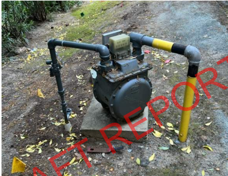
No seismic safety valve at gas meter.
