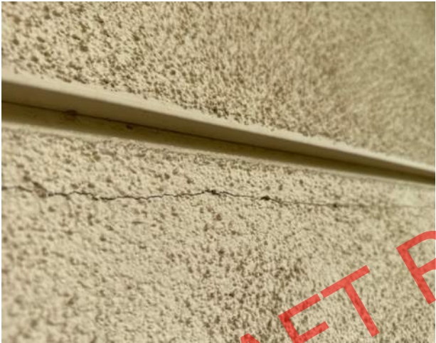
Crack under stucco reveal. 4102_NBL01_093
