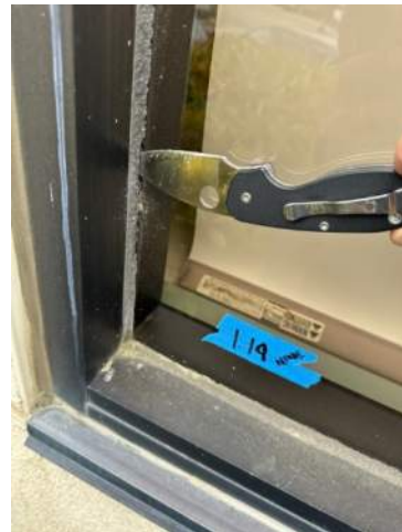
Window 1.19 – failure of wet-set sealant at glazing. Knife blade penetrates approx. 5/8" at gap in sealant.
