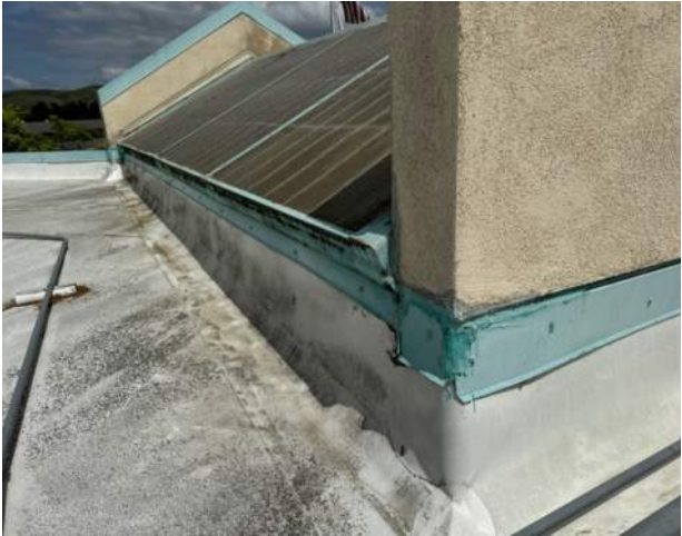
Remedial sealant repair attempts at skylight perimeter.
