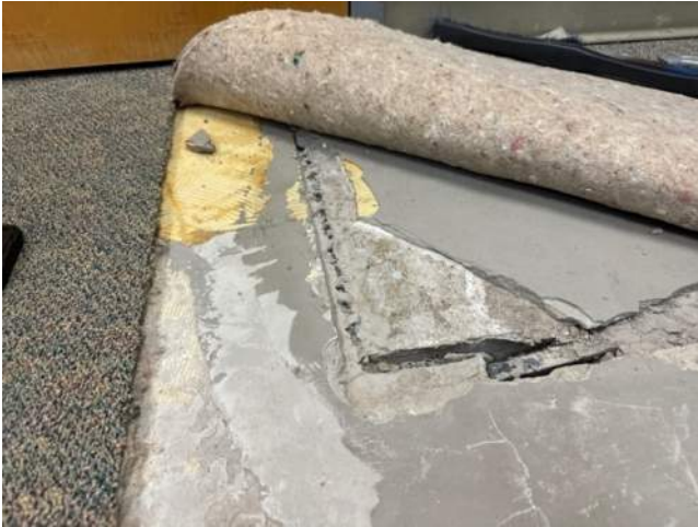
Evidence of various floor coverings installed & removed over time.
