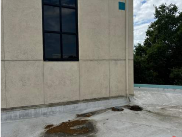
Low Roof - Insufficient sloping and drains at high point – near Window 2.25. 4102_NBL01_335
