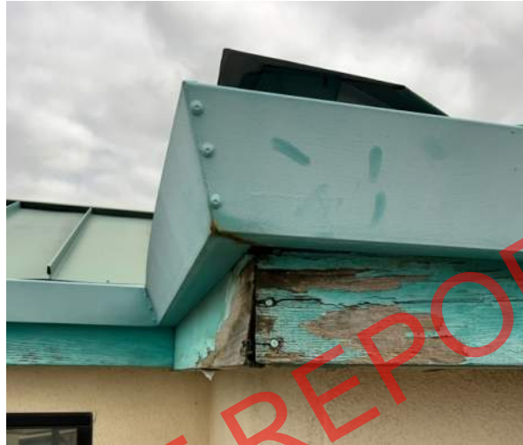
Rotted Wood Fascia. 4102_GEP01_054
