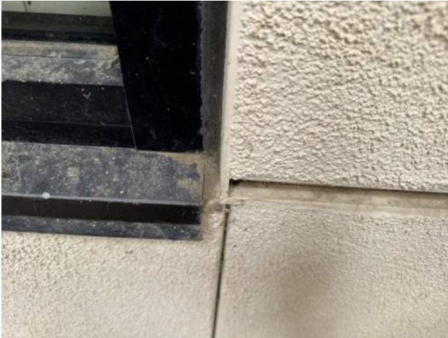
Window 1.16 – Cracked sealant at joint. 4102_NBL01_151
