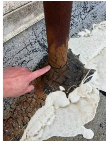
Gaps at sealed roof penetrations. 4102_GEP01_052
