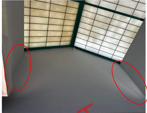
Staining at interior atrium at skylight corners.
