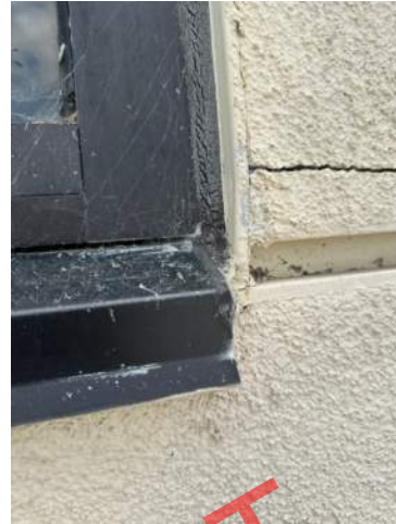
Window 2.15 – Cracked sealant at joint. 4102_NBL01_230
